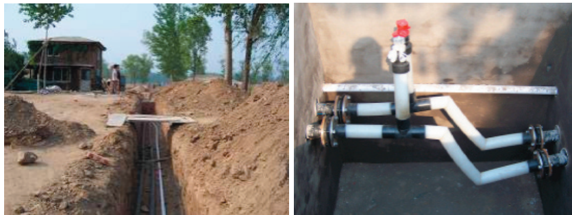
Fig. 7 Vacuum outdoors' pipelines and a vacuum lifting tank
